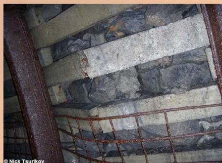
Wall cracks in an underground mine
